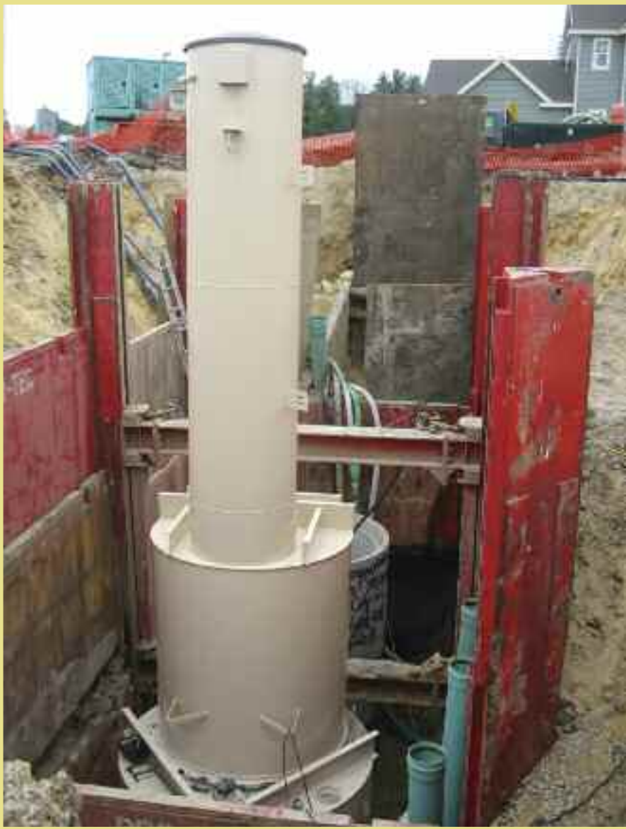
Hidden Oaks Lift Station — Middleton, WI
