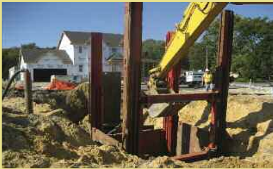
Hidden Oaks Lift Station — Middleton, WI
