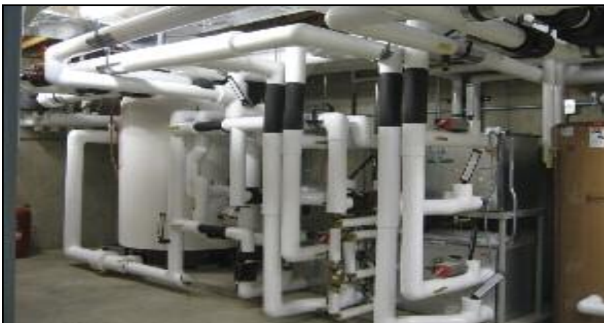
Heat pumps at the Aldo Leopold Legacy Center in Baraboo.
