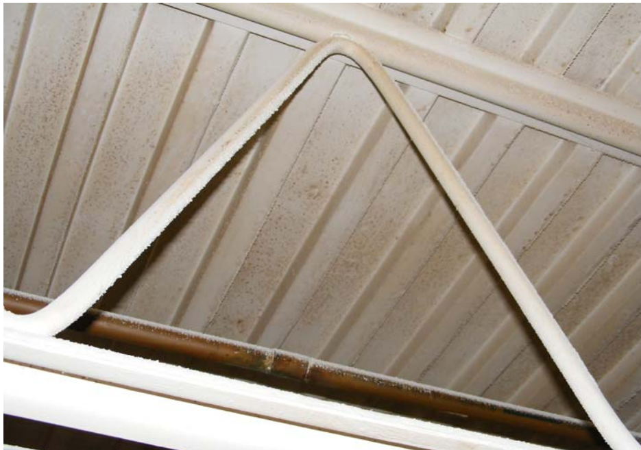
Combustible dust clings to surfaces such as these steel joists.
