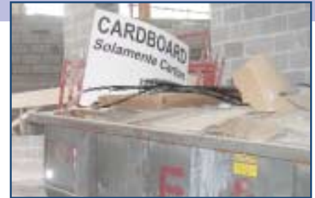
Recycling bins on location at AGC's new headquarters which is currently under construction.
